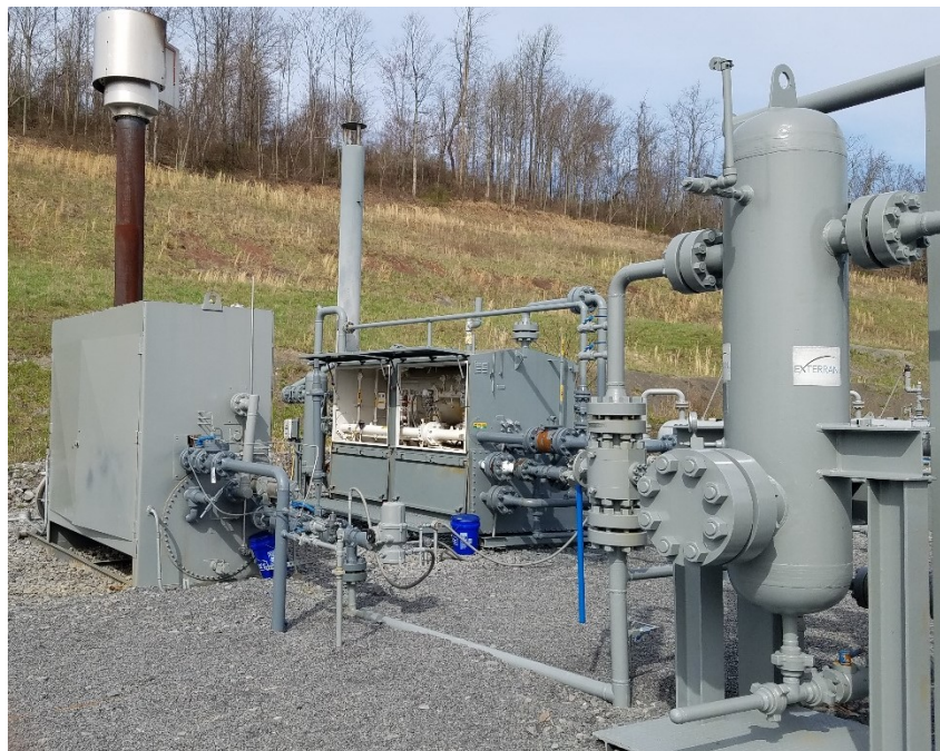
Figure 5.2. Natural Gas Burners and Other On-site Equipment
