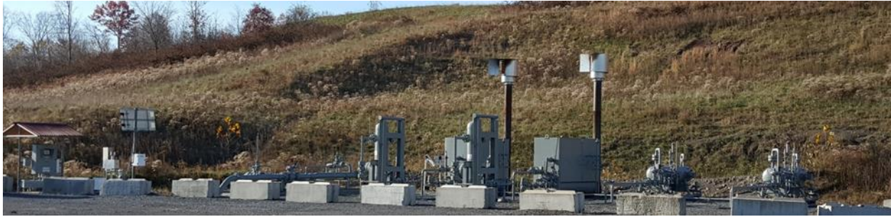
Figure 5.b.3: Natural Gas Burners and Other On-site Equipment
