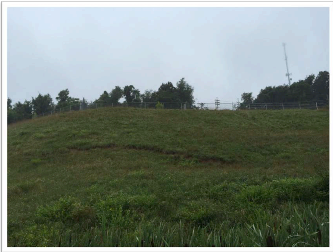
Figure 1. Scarp below Compressor Pad
